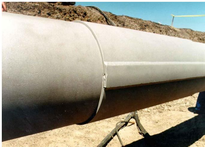
Fig. (6. 6) Example of installed and sandblasted steel compression sleeve (photograph Courtesy of Petro-Line, Inc.).
