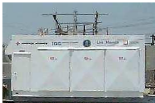
Fig (4.5) The General Atomics/Intermagetics General superconducting Fault Current Controller, employing HTS superconductors.
