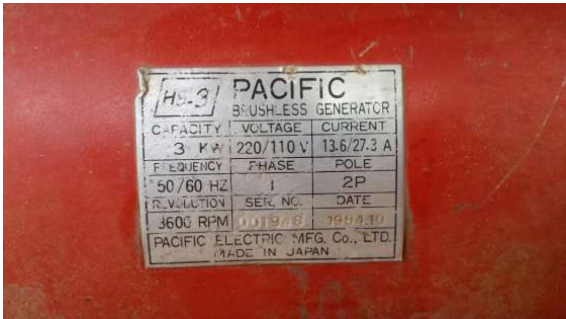
Figure 3.3: brushless Synchronous generator nameplate.
