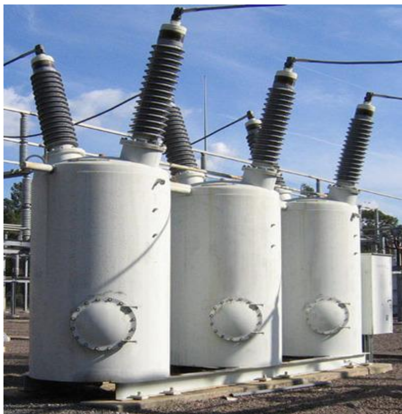
Figure (2-2): Oil circuit breaker
