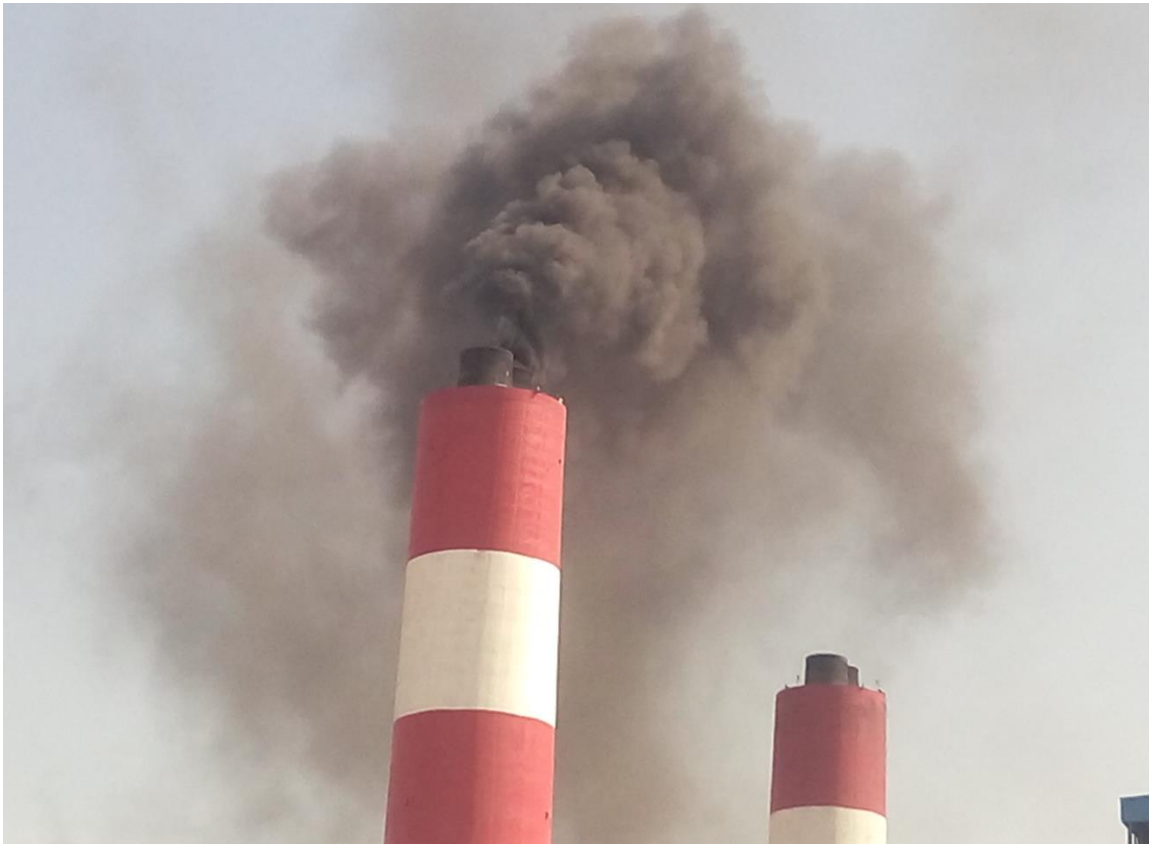
Figure ( 2- 16) boiler bad firing exhaust
