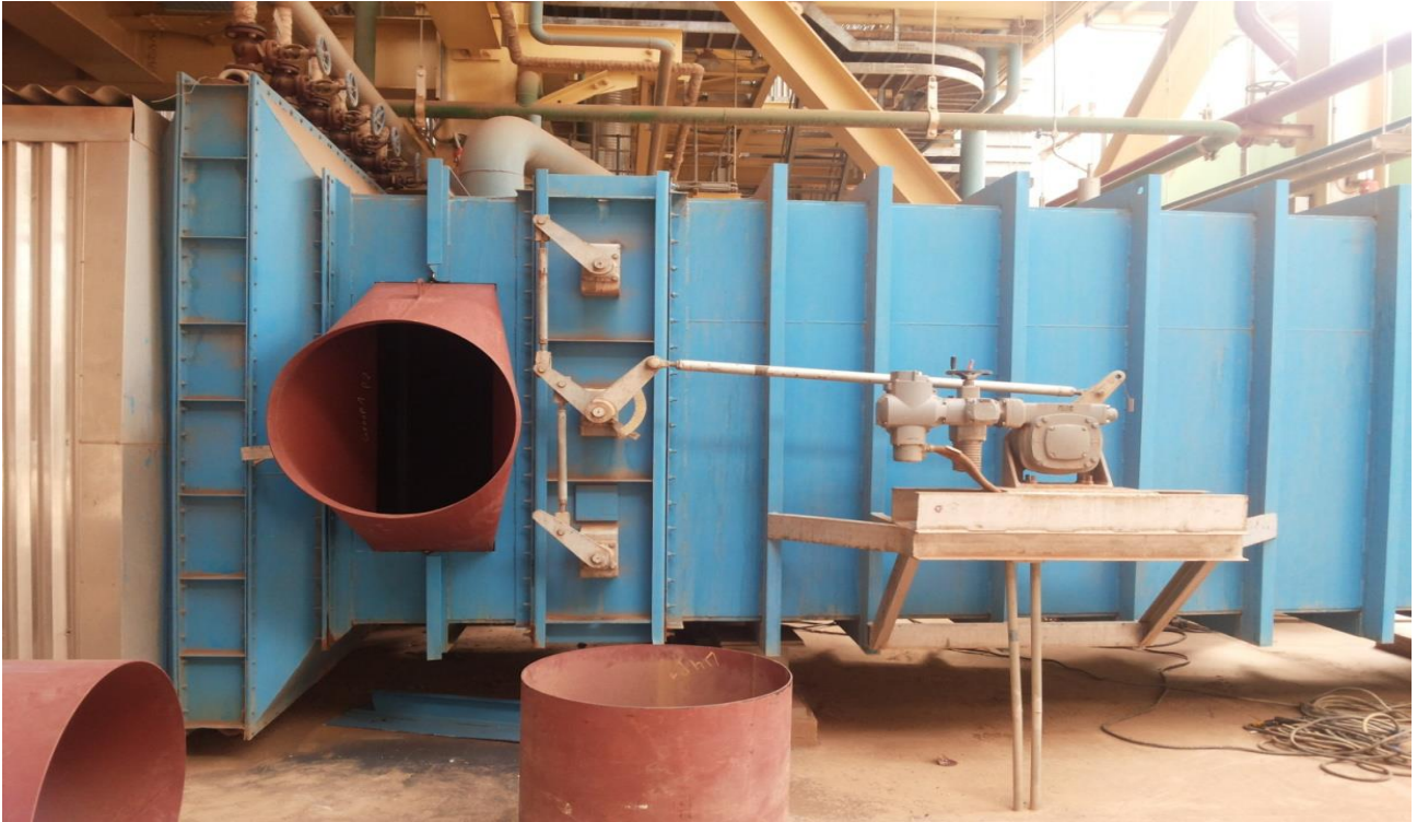
Figure (3 -2b) PA duct start from DF Fan downstream
