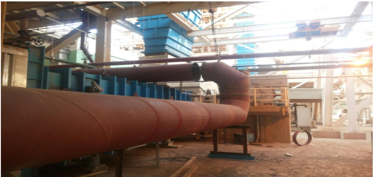
Figure (3 -2c) PA duct to PA fans as build
