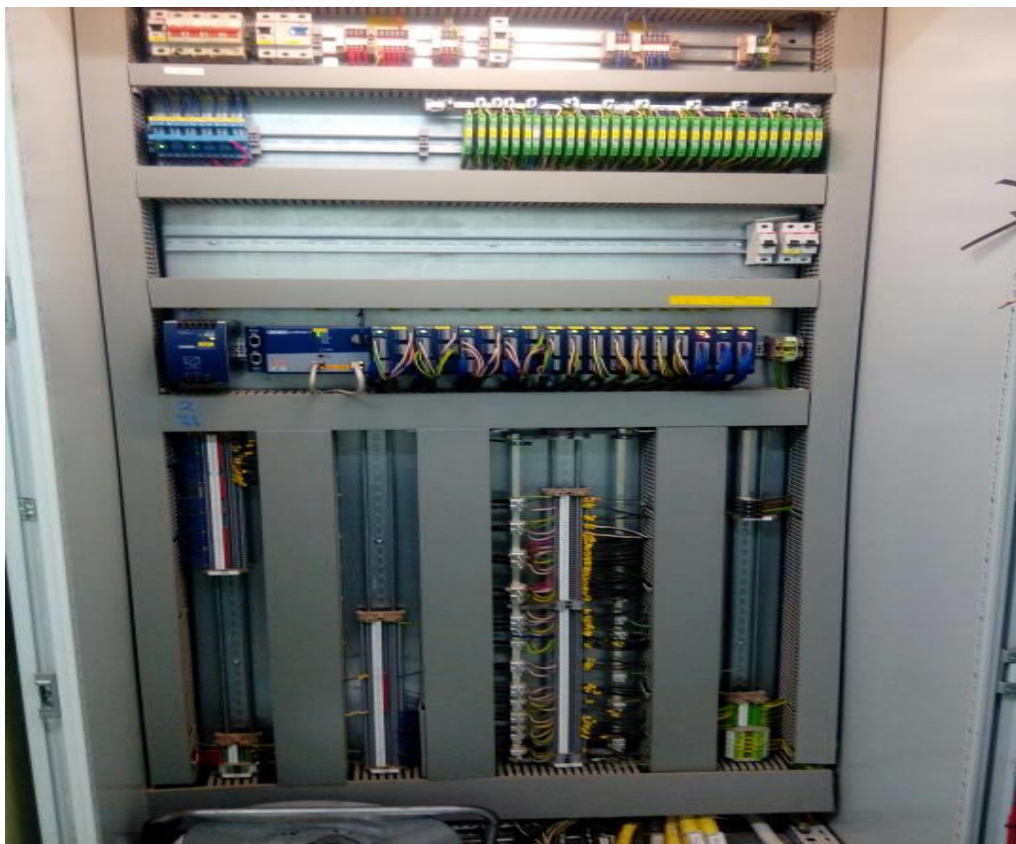
Figure ( 3- 6) Electrical control Panel
