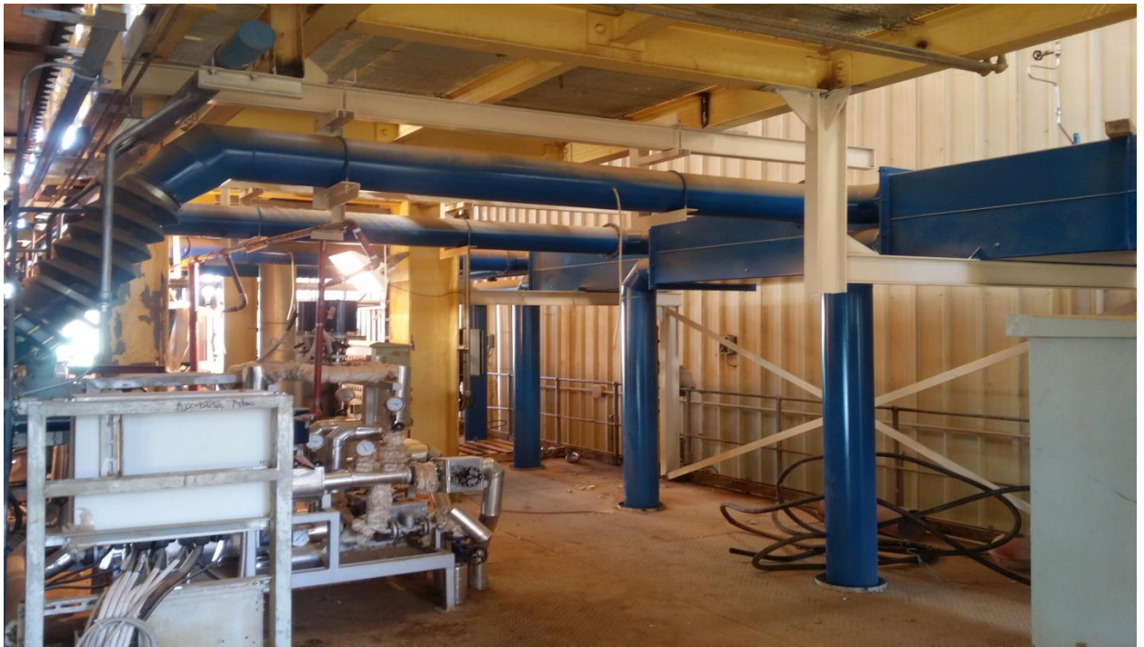
Figure (3 – 2e) duct distributing to burners as build
