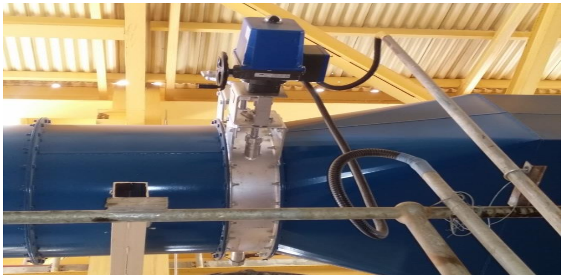
Figure (3-4) P A control damper
