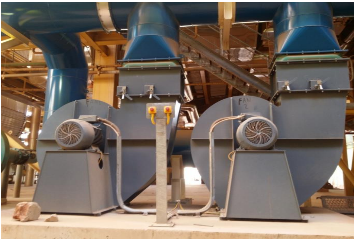
Figure (3-3b) PA fans and Bypass damper as build
