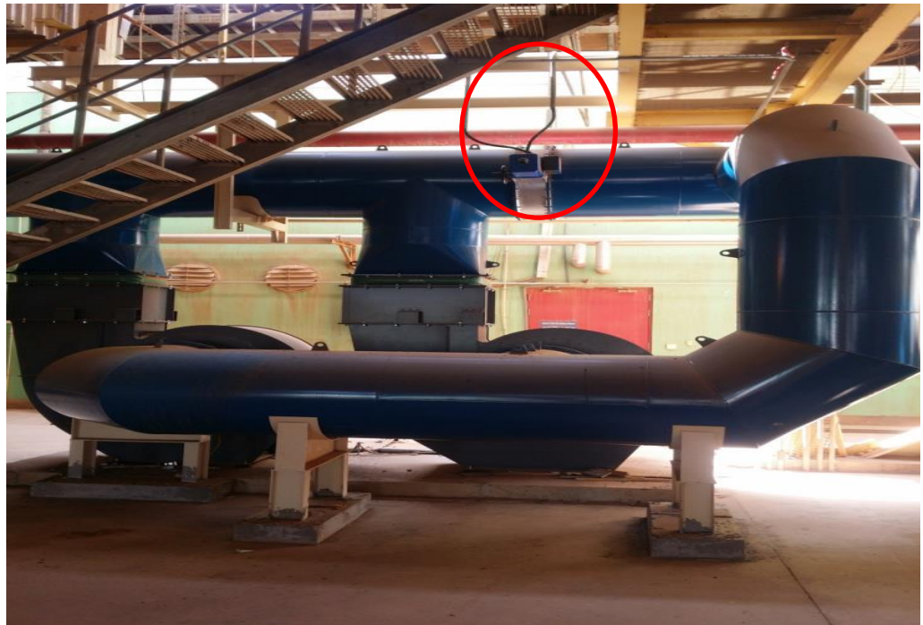
Figure (3-3c) PA Bypass damper
