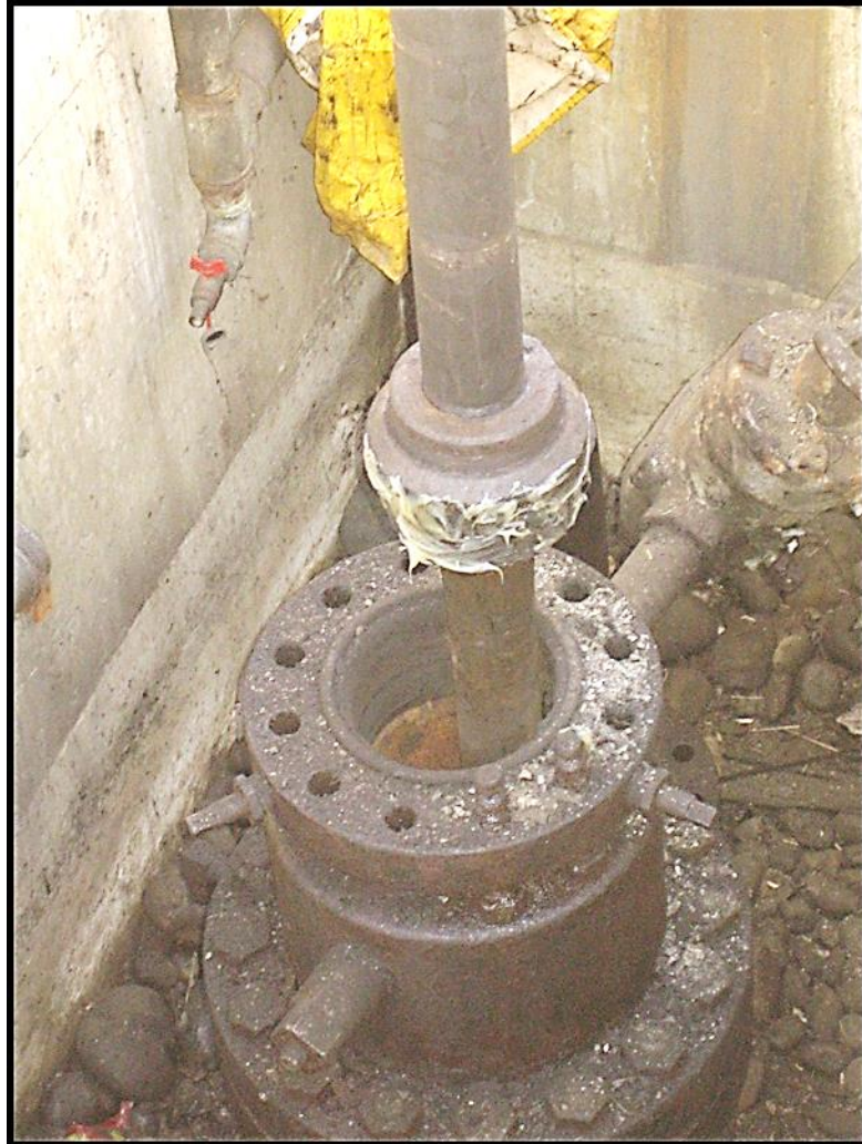
Figure (2. 10) setting torque anchor (PCM MOINEAU OILFIELD)
