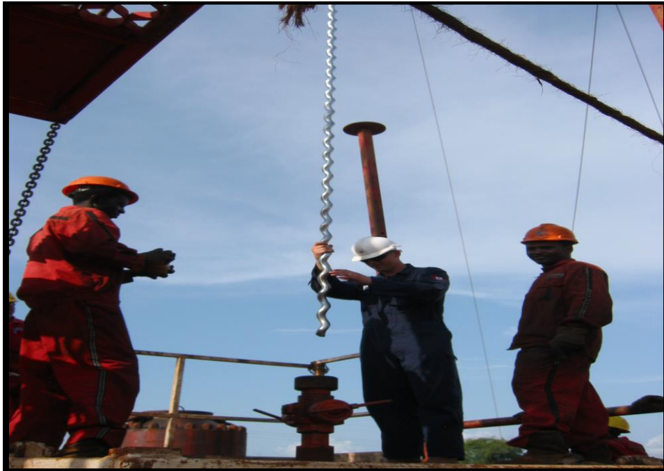
Figure (2. 12) running rotor in hole (PCM MOINEAU OILFIELD)
