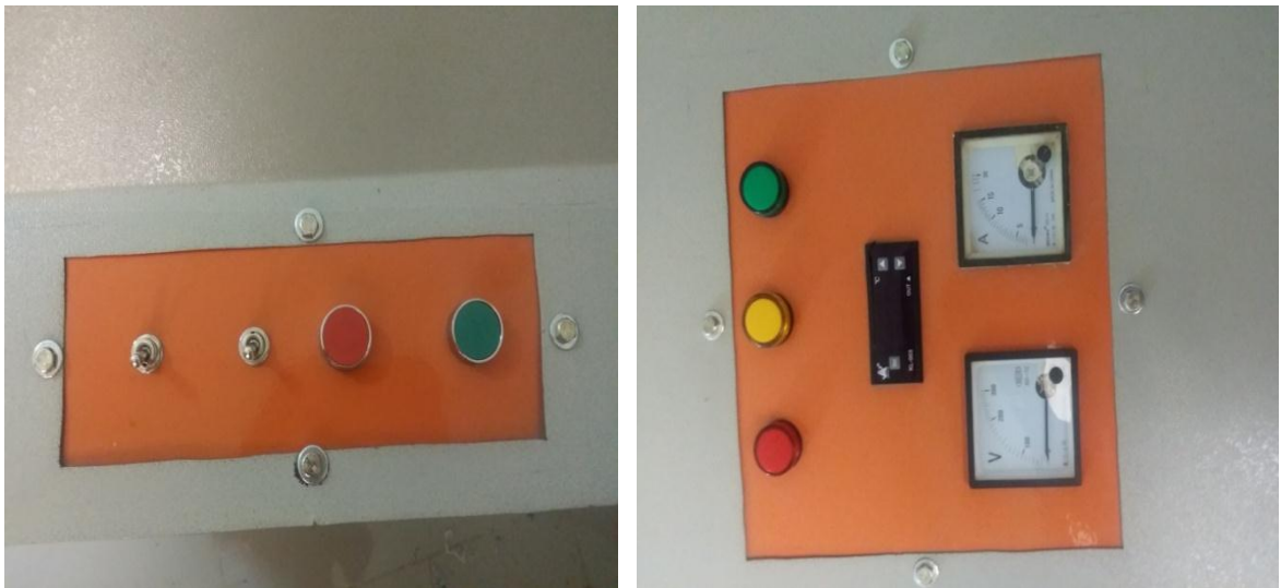
Figure (2.10): The interface unit
