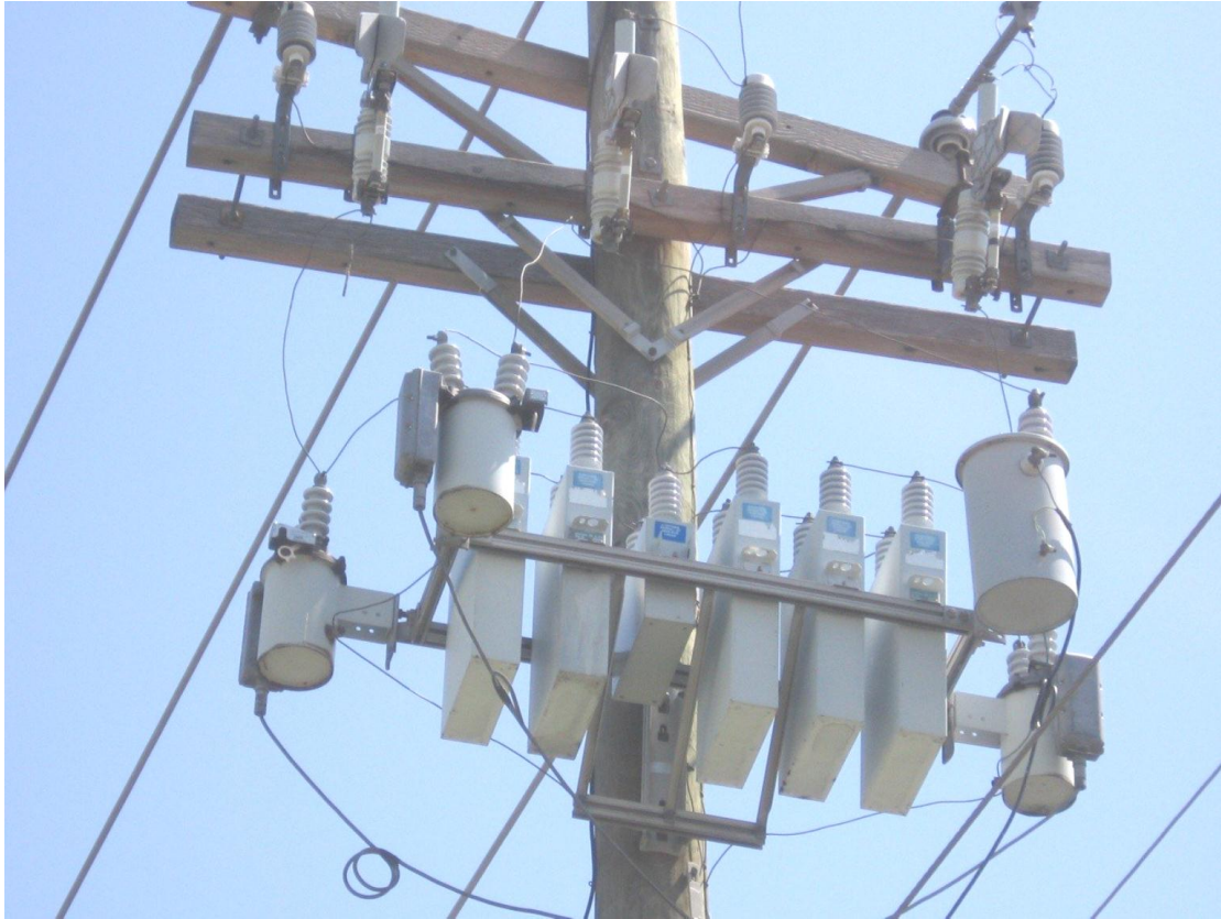
Figure A. 1 Line Mounted Capacitor Bank
