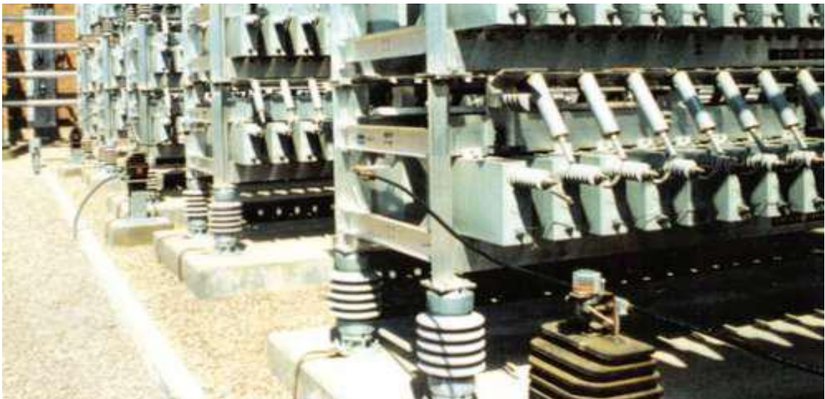
Figure A. 2 Capacitor bank (externally fused)
