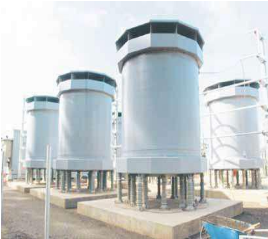
Figure A. 4 SVC Units
