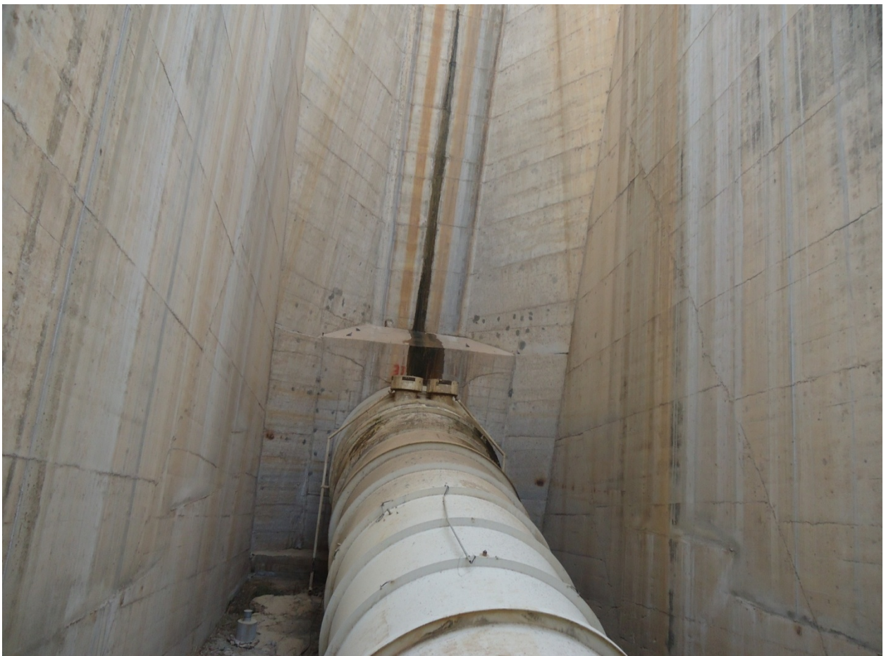
Figure (2.3) The Penstock
