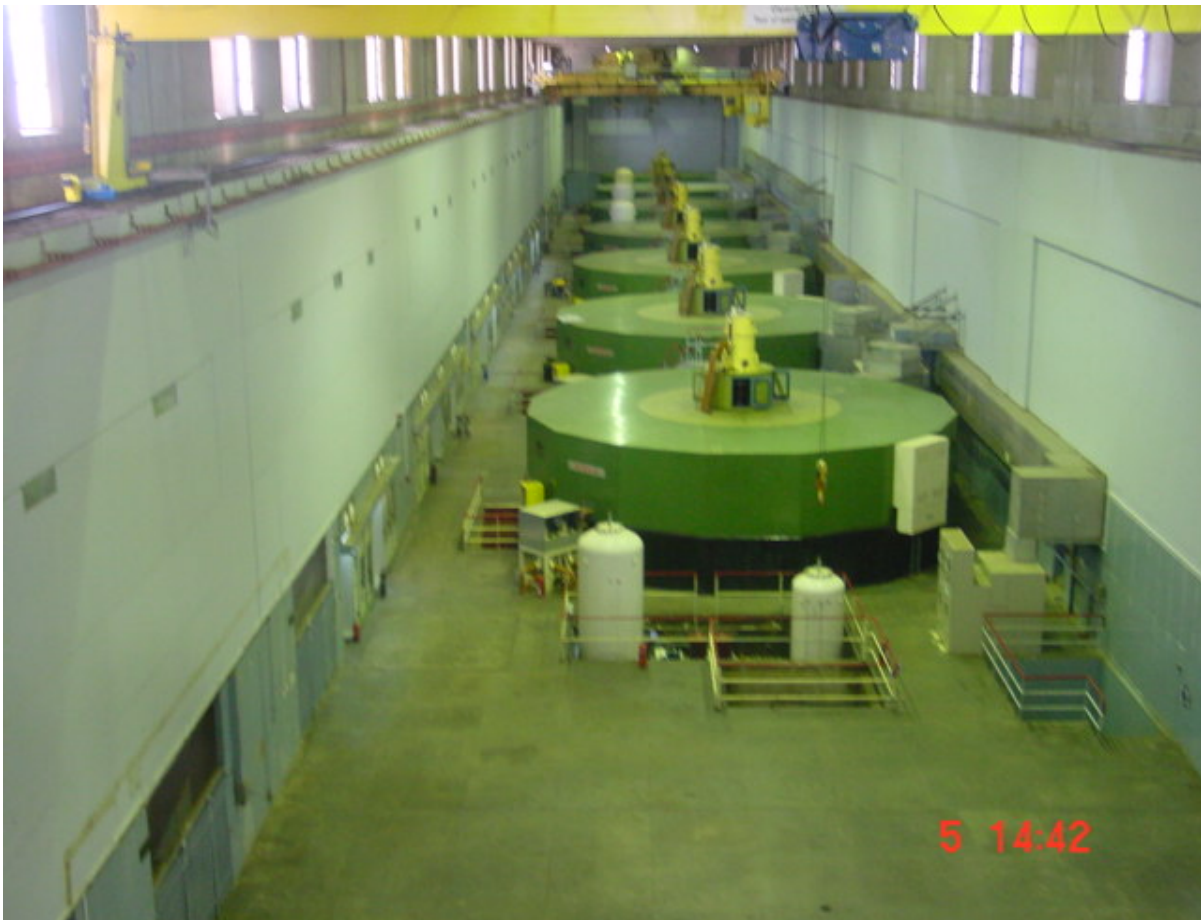
Figure (2.8) The Generator
