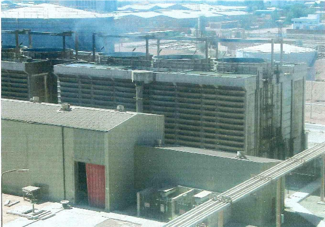
Figure (2-6) cooling tower with cooling fans [6]
