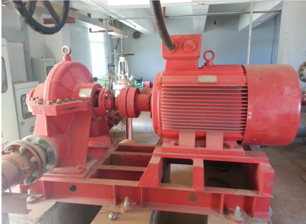
Figure 3.5: Main Electric Pump.
