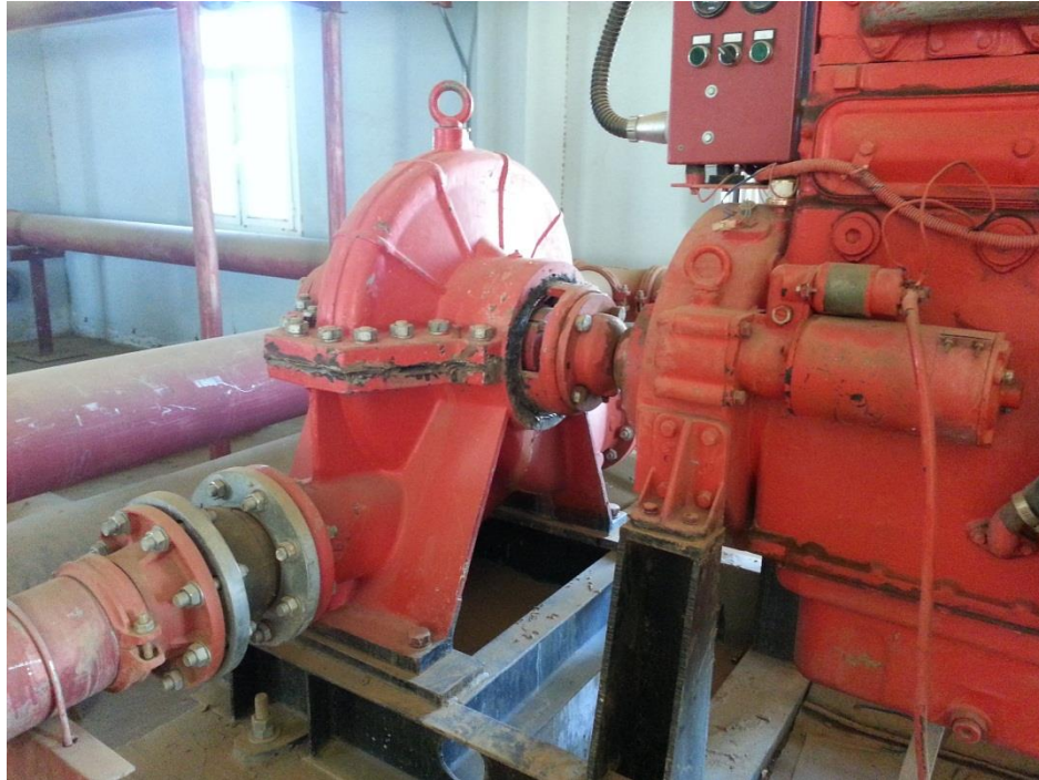
Figure 3.12: Pump Connected to Diesel Engine.
