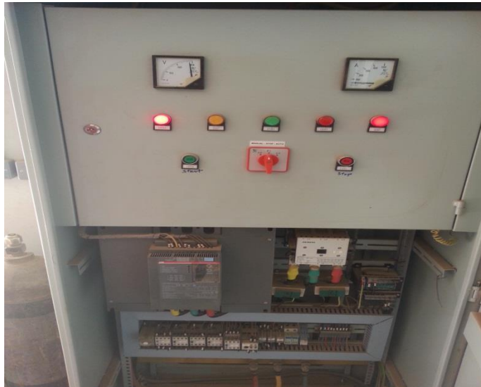
Figure 2.6: Electric Motor Controller
