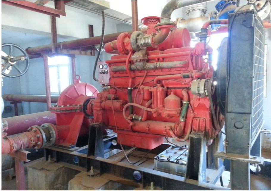
Figure 3.6: Diesel Engine Pump.
