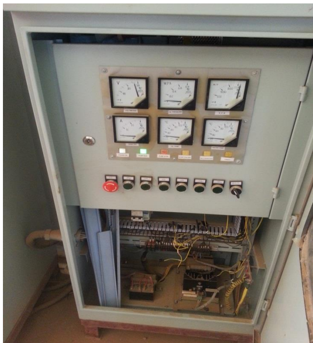
Figure 2.7: Diesel Engine Controller.
