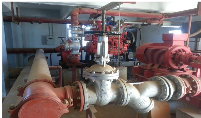
Figure 3.1: Fire Pumps Room.
