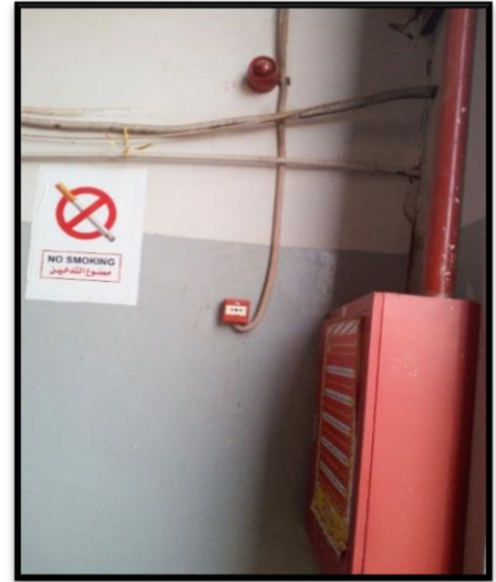
B. Manual alarm system in factory.
