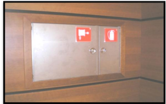
The Figure (3-17) shows manual fire extinguishers S: www.arabicsafety.com
