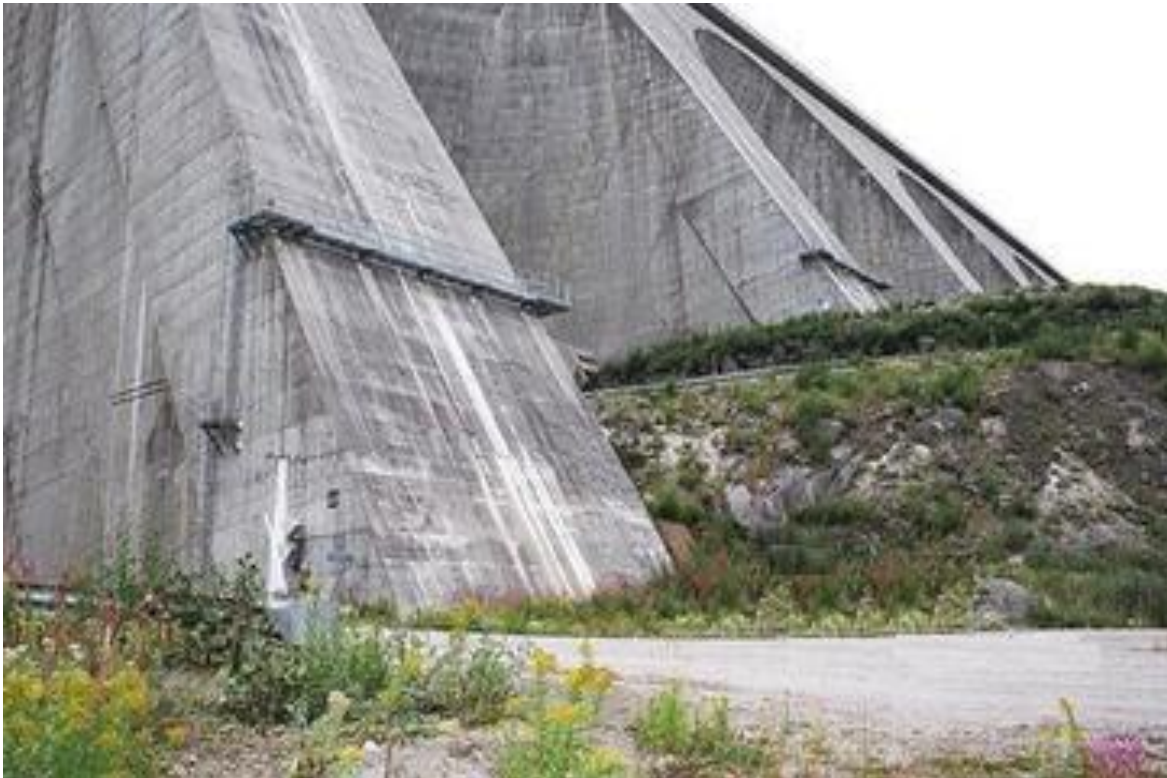
Fig.No.(2.9):One of the Buttresses in the Manic-Ceng Buttress Dam in Québec, Canada ( www.dappolonia.com ).
