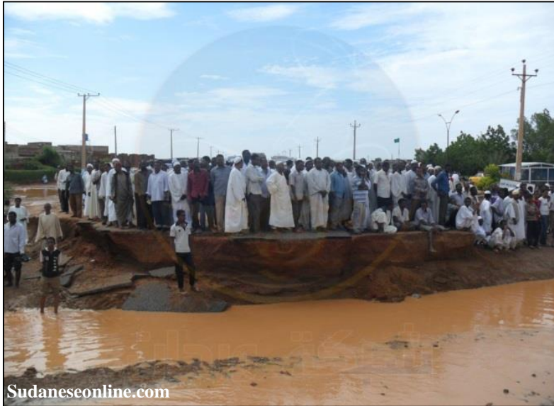
Figure 1.4 Washed away Highways
