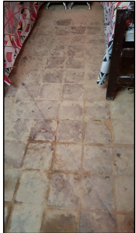
(0.15x0.15) m Cement tiles (Bedroom)
