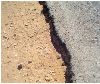
Fig. A.23: Medium Severity Lane/Shoulder Drop-off
