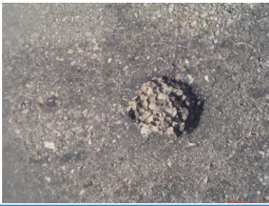
Figure A.32 Low Severity Potholes
