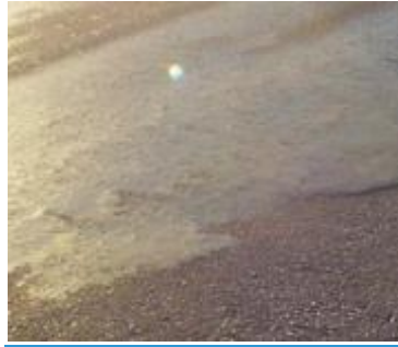
Fig. A.6: High Severity Bleeding
