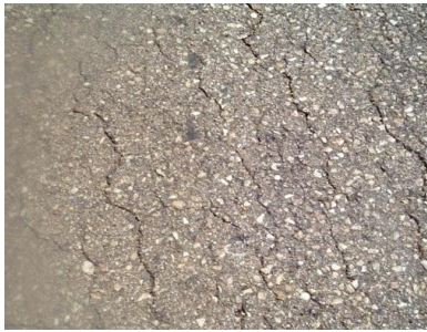
Fig. A.2: Medium Severity Alligator Cracking
