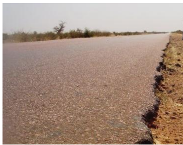
Fig. A.24: High Severity Lane/Shoulder Drop-off
