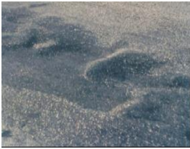
Figure A.44 Low Severity shoving
