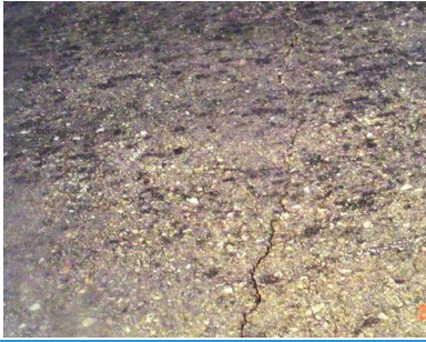
Figure A.38 low Severity reflection crack
