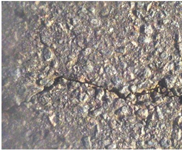
Fig. A.26: Medium Severity Longitudinal & Transverse Cracks
