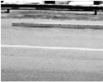
Fig. A.14: Medium Severity Corrugation
