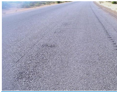
Figure A.35 Low Severity Raveling
