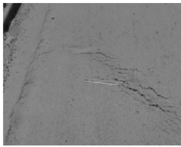
Figure A.48 Medium Severity Slippage Cracks
