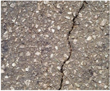
Figure A.39 medium Severity reflection cracks
