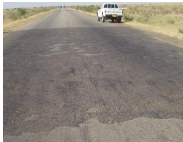
Fig. A.30: High Severity Patching
