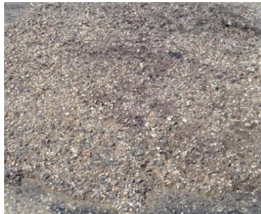
Figure A.36 Medium Severity Raveling
