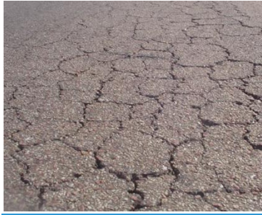
Fig. A.3: High Severity Alligator Cracking
