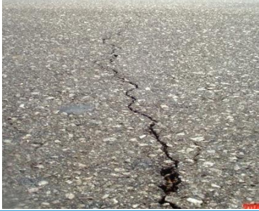
Figure A.40 High Severity reflection cracks
