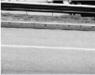
Fig. A.13: Low Severity Corrugation
