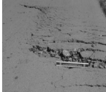
Figure A.49 High Severity Slippage Crack
