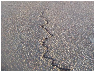
Fig. A.27: High Severity Longitudinal & Transverse Cracks
