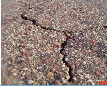
Fig.A.9: High Severity Block Cracking
