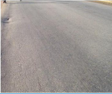
Figure A2.41 low Severity Rutting
