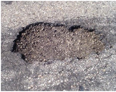
Figure A.33 Medium Severity Potholes
