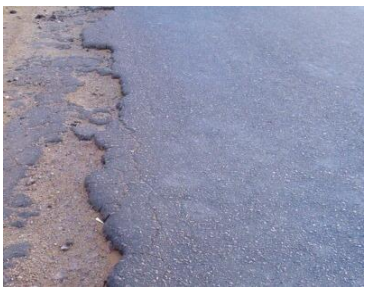
Fig. A.21: High Severity Edge Cracking
