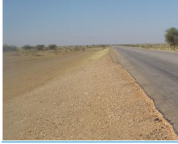
Fig. A.22: Low Severity Lane/Shoulder drop-off
