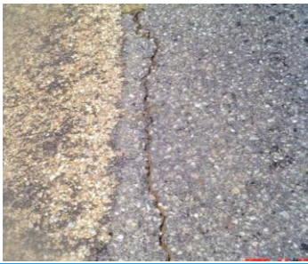
Fig.A.20: Medium Severity Edge Cracking
