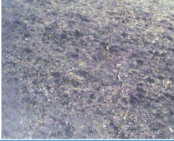
Fig. A.25: Low Severity Longitudinal & Transverse Cracks
