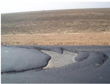
Figure A.45 Medium Severity shoving
