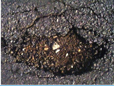
Figure A.34 High Severity Potholes
