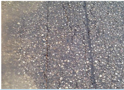
Fig. A.1: Low Severity Alligator Cracking
