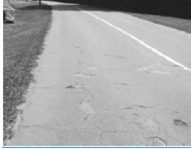
Figure A.37 High Severity Raveling
