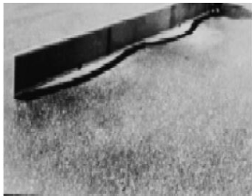
Fig. A.15: High Severity Corrugation
