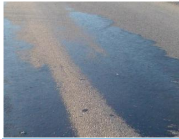
Fig. A.5: Medium Severity Bleeding
