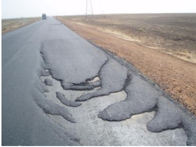
Figure A.46 high Severity shoving
