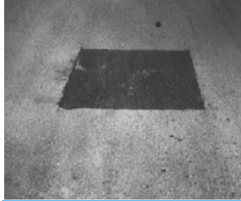
Fig. A.28: Low Severity Patching
