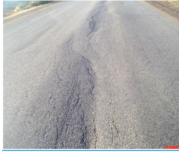
Fig. 2.12: High Severity Upheavals and Settlements
