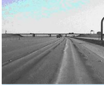
Figure A.43 High Severity Rutting
