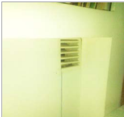
Fig.4.51 Wind catcher outlet in guest room .
