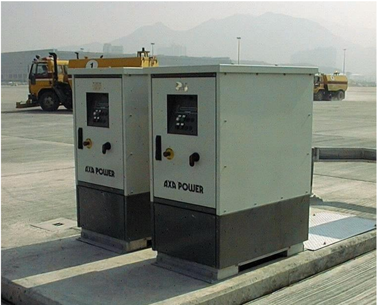
Figure 2.2: Two 90 kVA point of use frequency converters
