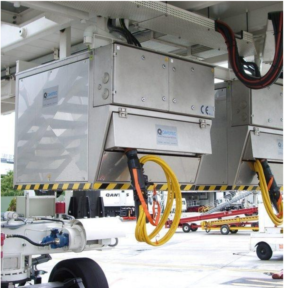
Figure 2.3: Bridge Mounted Cable Coiler
