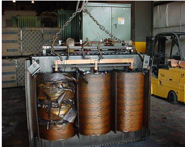
Fig 2.2- Power transformer failure
