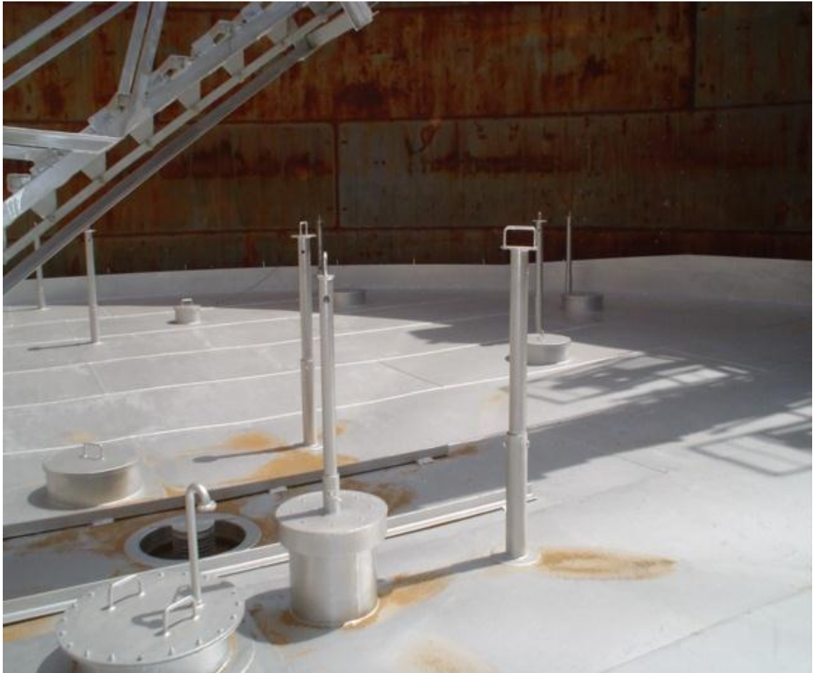
Fig:2.3. floating roof tank
