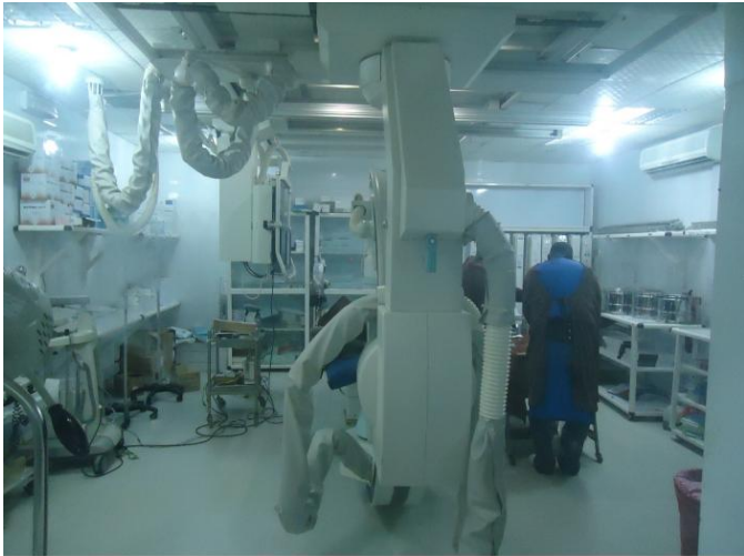
Fig 3-7: Machine(cath-lab in Alshaab hospital)
