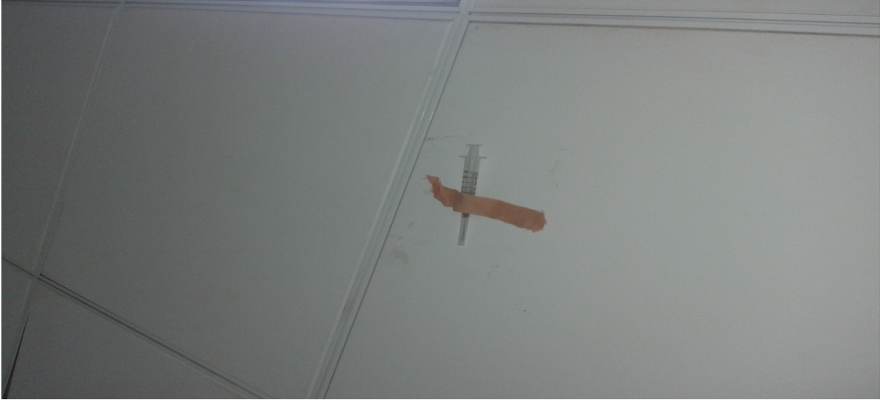
Figure 3-34: image shows the point source centering over the camera head at ceiling
