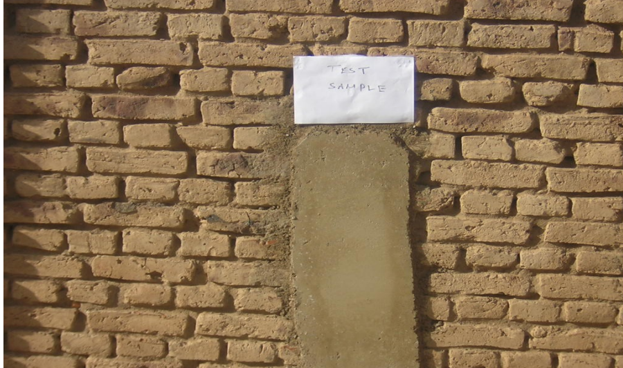
Plate C6: Wall plaster Strip (test sample)
