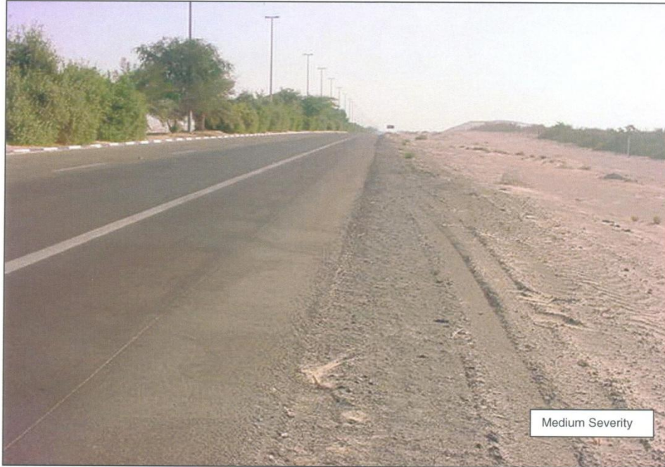
Photo 2: Lane/Shoulder Drop off (Distress Type 9)
