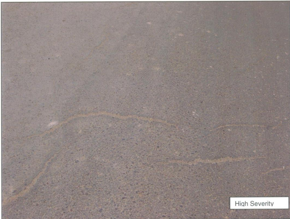
Photo 3: Slippage Cracking (Distress Type 17)
