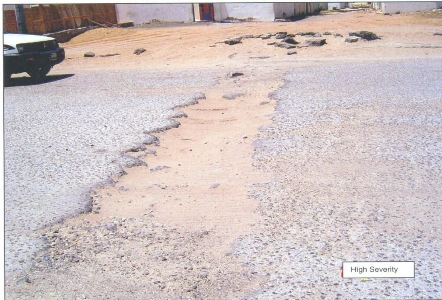
Photo 3: Patching & Utility Cut Patching (Distress Type 11)
