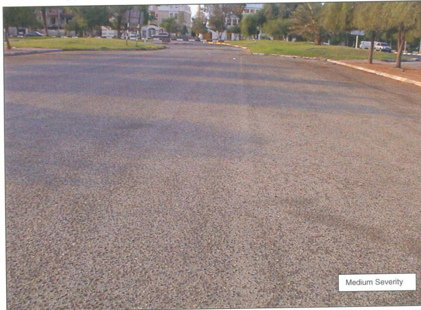
Photo 2: Rutting (Distress Type 15)
