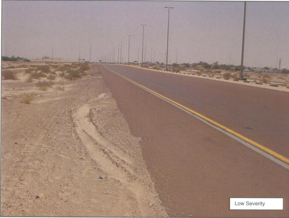
Photo 1: Lane/Shoulder Drop off (Distress Type 9)
