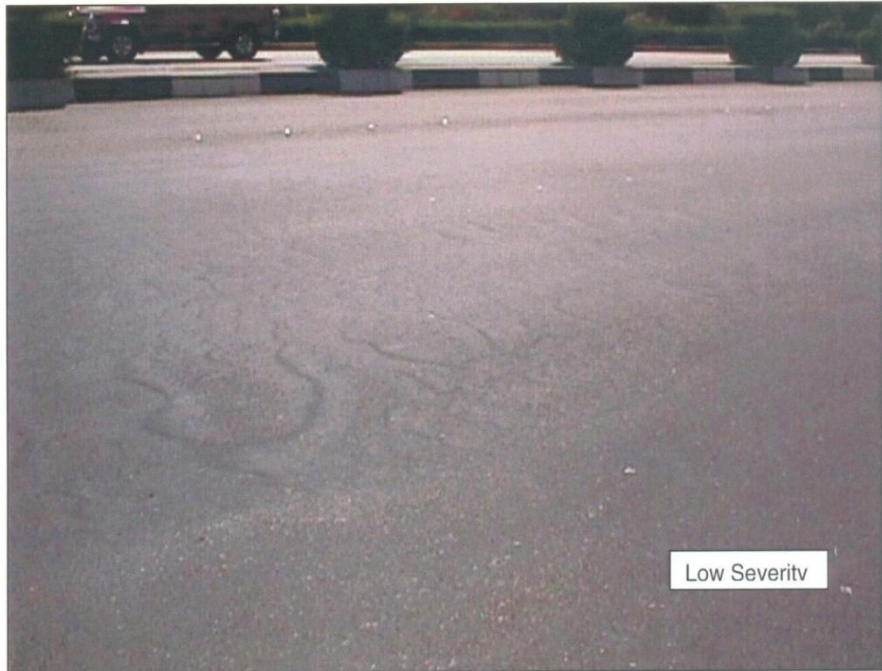
Photo 1: Shoving (Distress Type 16)
