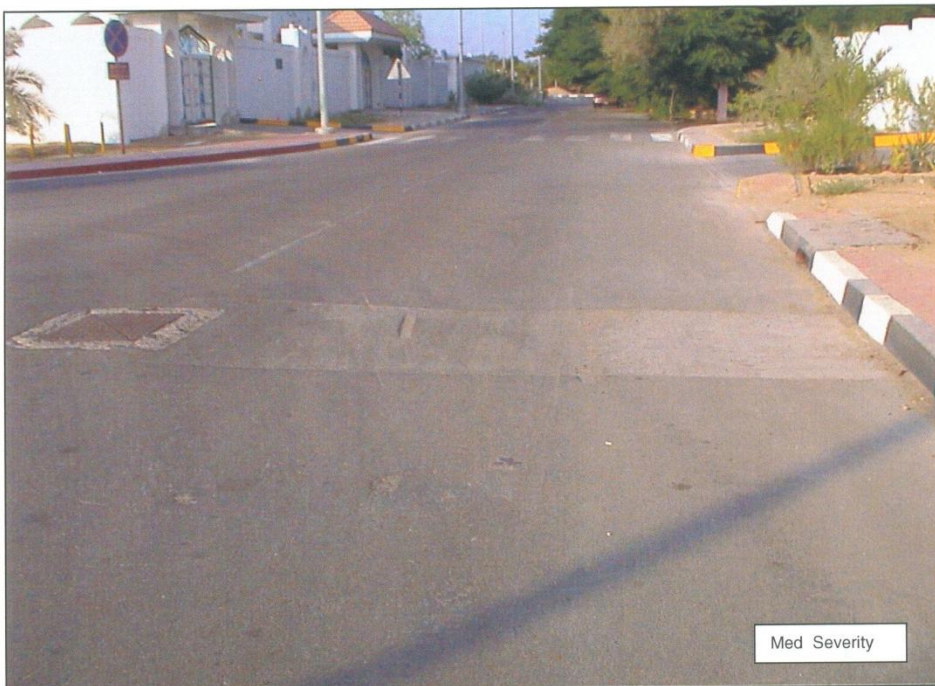
Photo 2: Patching and Utility Cut Patching (Distress Type 11)
