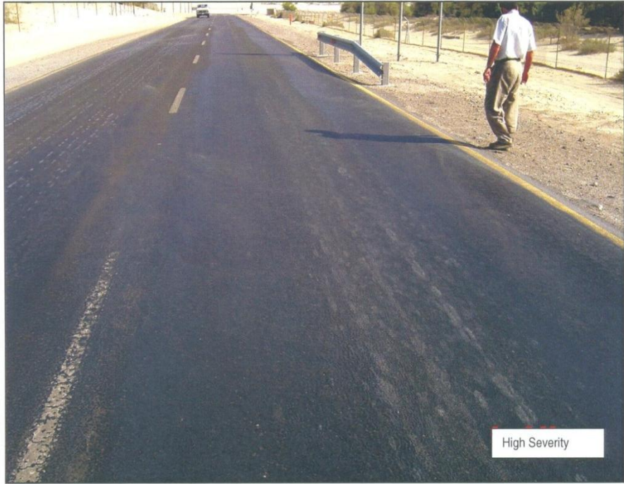
Photo 3: Bleeding (Distress Type 2)
