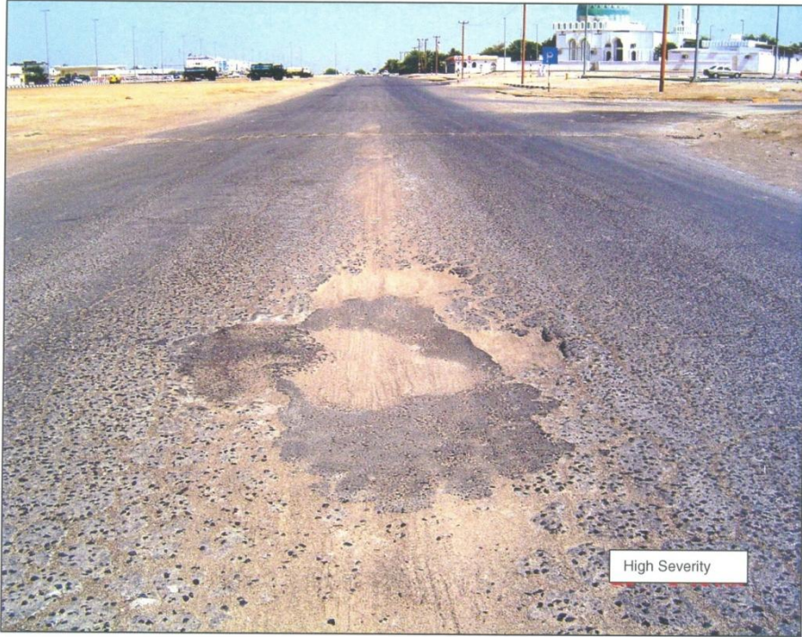
Photo 3: Pothole (Distress Type 13).
