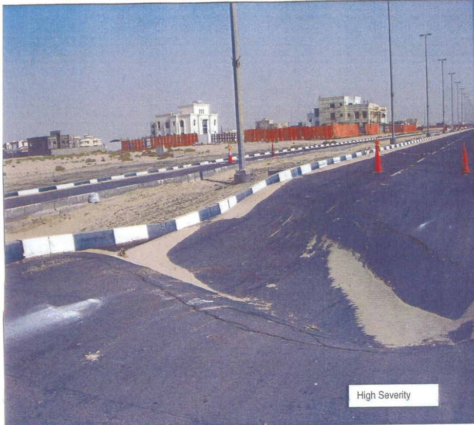
Photo 3: Depression (Distress Type 6)
