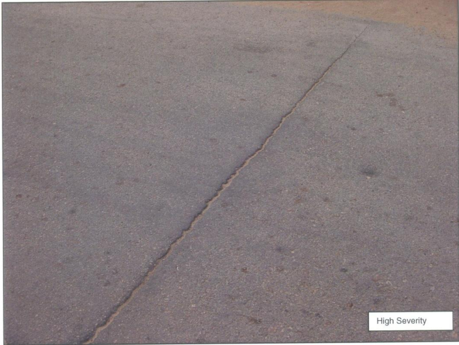
Photo 3: Joint Reflection (Distress Type 8)
