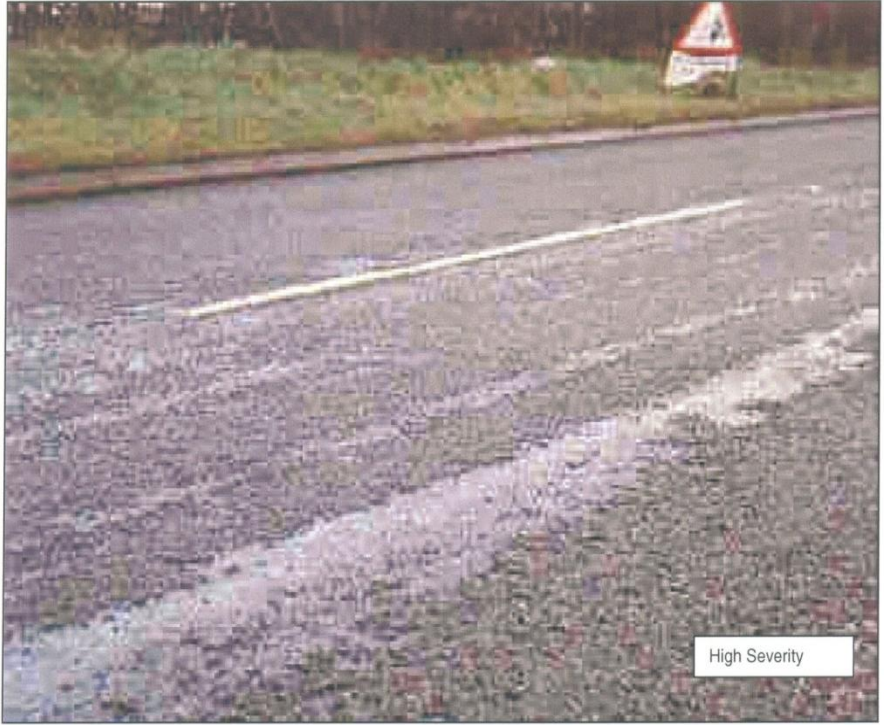
Photo 4: Bleeding (Distress Type 2)
