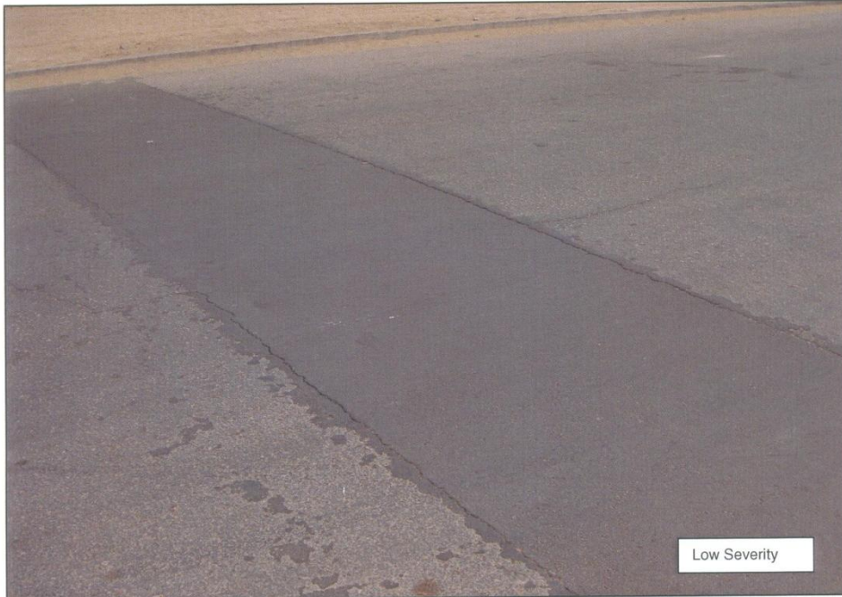
Photo 1: Patching and Utility Cut Patching (Distress Type 11).
