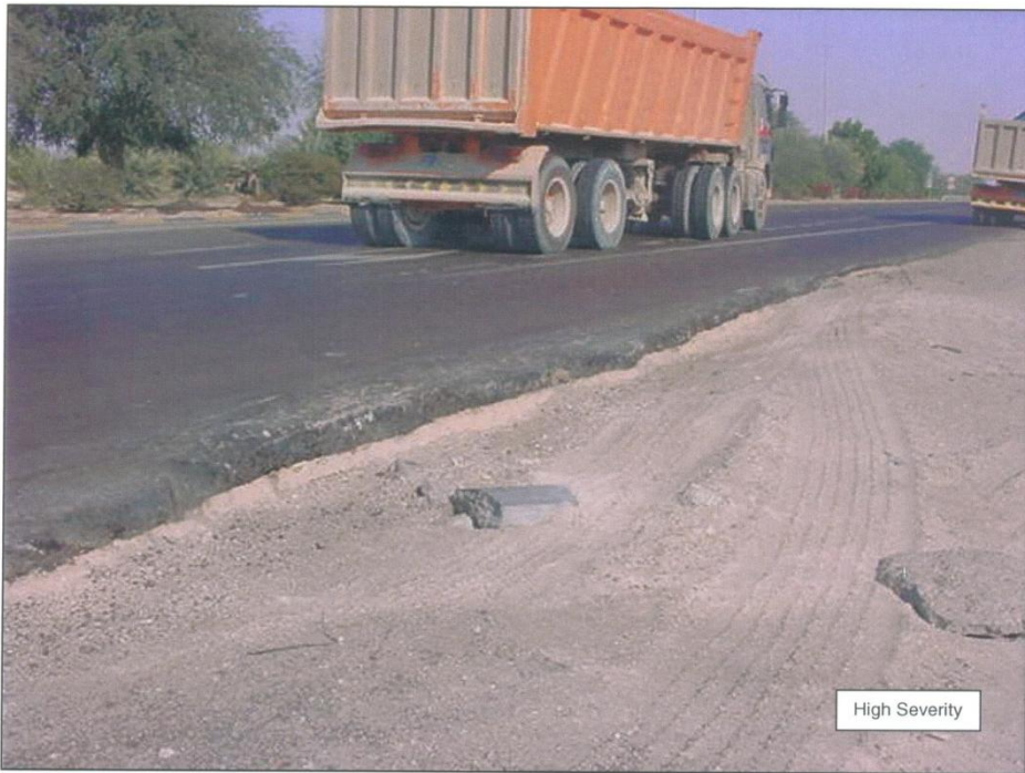
Photo 3: Lane/Shoulder Drop off (Distress Type 9)
