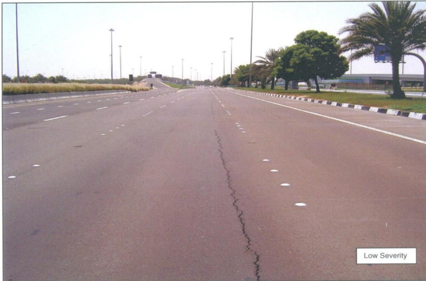
Photo 1 : Longitudinal & Transverse Cracks ( Distress Type 10)
