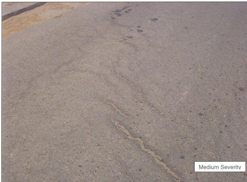
Photo 2: Slippage Cracking (Distress Type 17)
