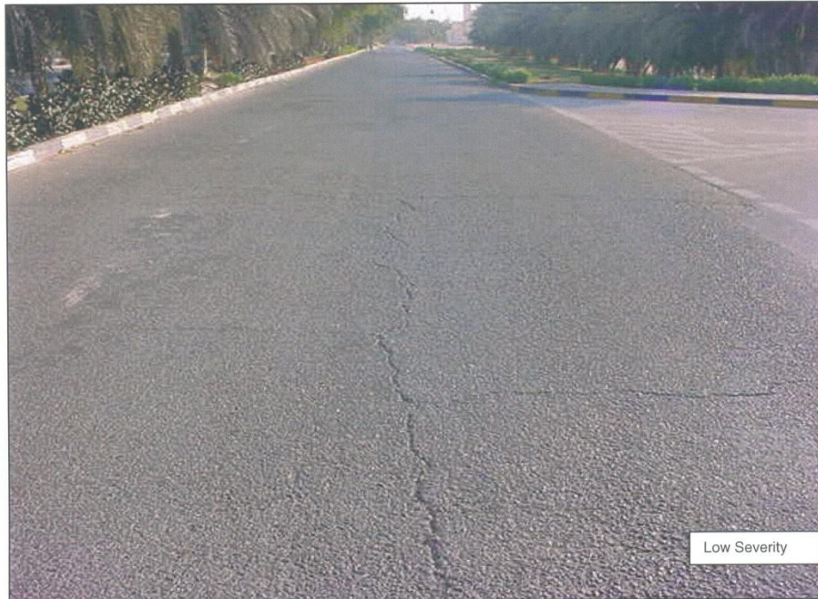
Photo 1: Block Cracking (Distress Type 3)
