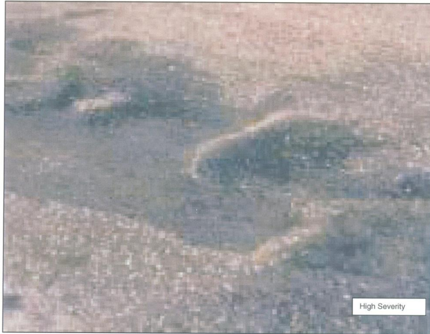
Photo 3: Shoving (Distress Type 16)
