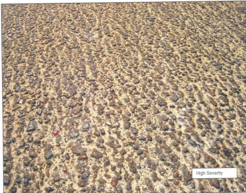
Photo 3: WEATHERING AND RAVELING (19)
