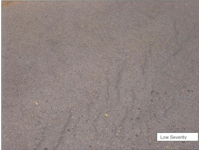
Photo 1: Slippage Cracking (Distress Type 17)
