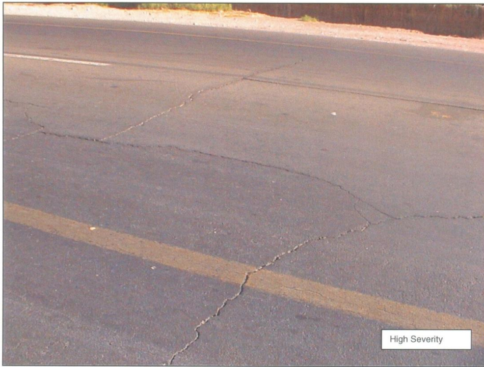
Photo 3: Block Cracking (Distress Type 3)
