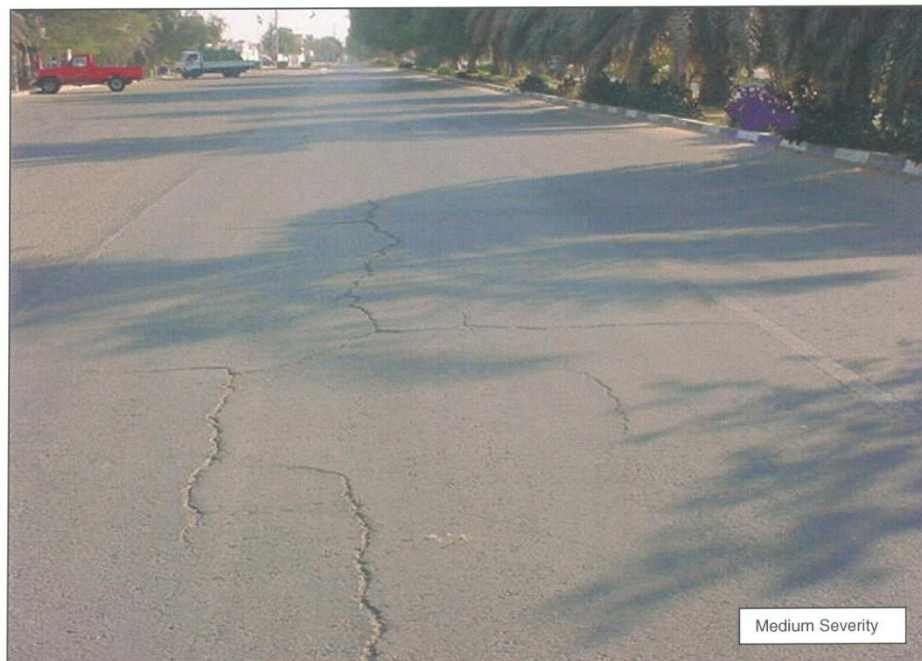
Photo 2: Block Cracking (Distress Type 3)
