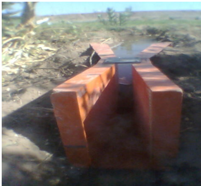
Plate 7: Parshall flume 2inch
