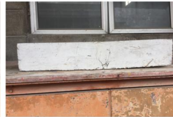
Prism failure (left view) – only cracks appeared
