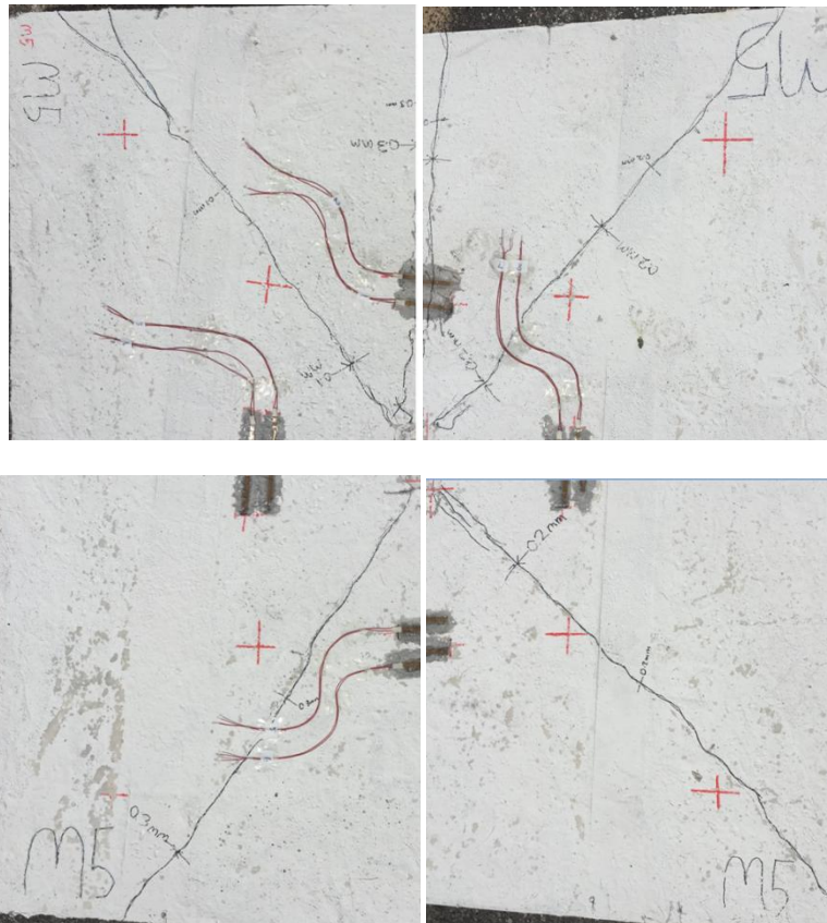
Figure B7: Failure for Slab Specimen M5 (2m drop) – another plan view (0.1, 0.2 and 0.3mm crack widths)
