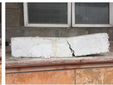
Prism failure (left view) – almost splitted into two sections
