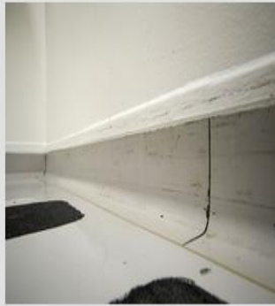
Image: Cracked joint
