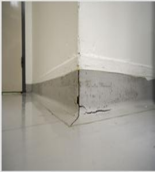
Image: Cracked joint
