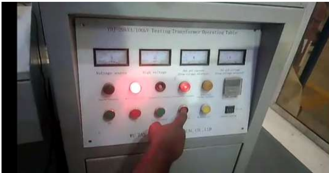
Figure 4.7: single phase 20KVA, 100KV transformer test unit
