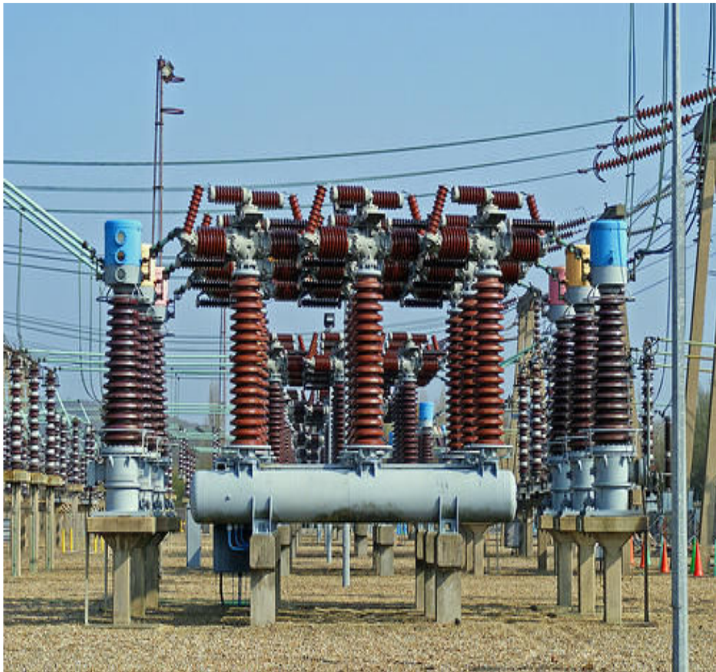
Figure 2.8: Air blast circuit-breakers
