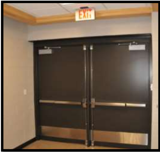
The figure (2-37) shows emergency exit door
