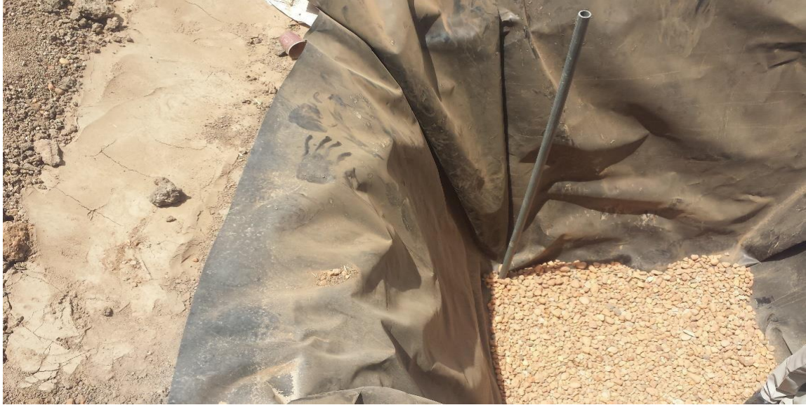
Fig (3.8) the leachate collection system
