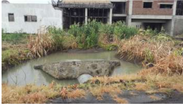
Figure 4.8 Accumulation of soils on the road and Edge of the road erosion
