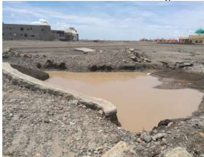
Figure 4.9 the side drain was blocked with soil, debris, vegetation, wheel and solid waste.
