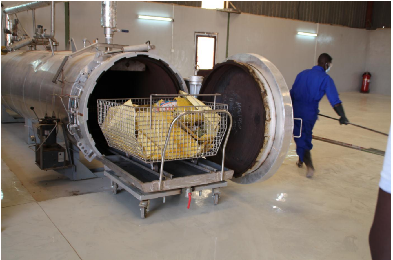
Photo D-7: Entering trolley of medical waste into Autoclave
