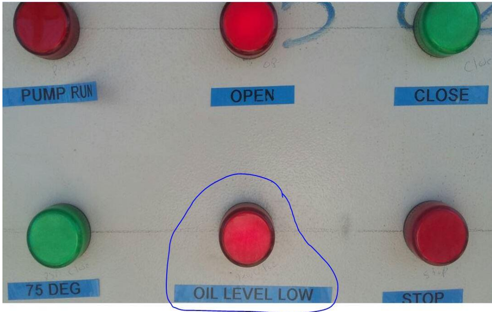
Figure 4.19: Hydraulic oil level low alarm
