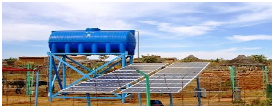
Figure1.1 solar pumping systems in Zamzam IDPs Camp
