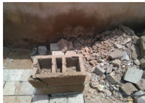
Fig 4.10 Crack in hollow concrete block
