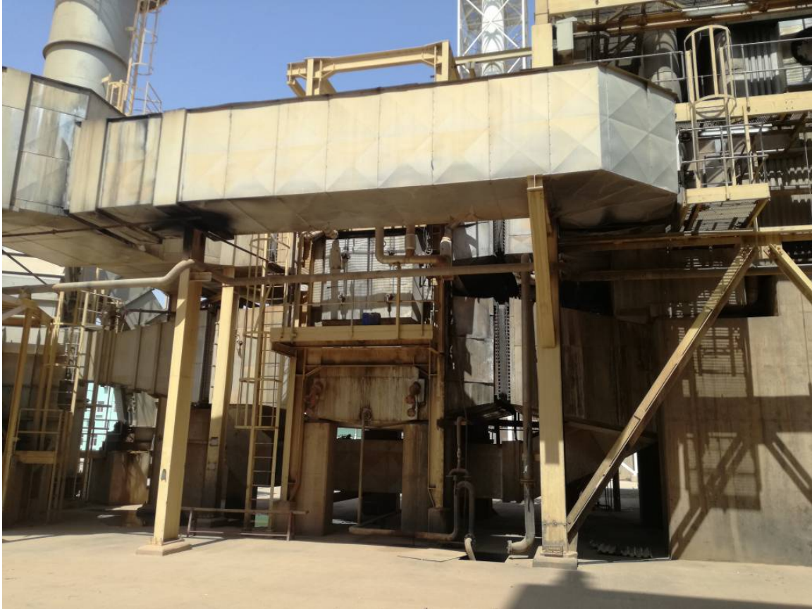
Fig (3 – 4) rotary Air Pre-heater
