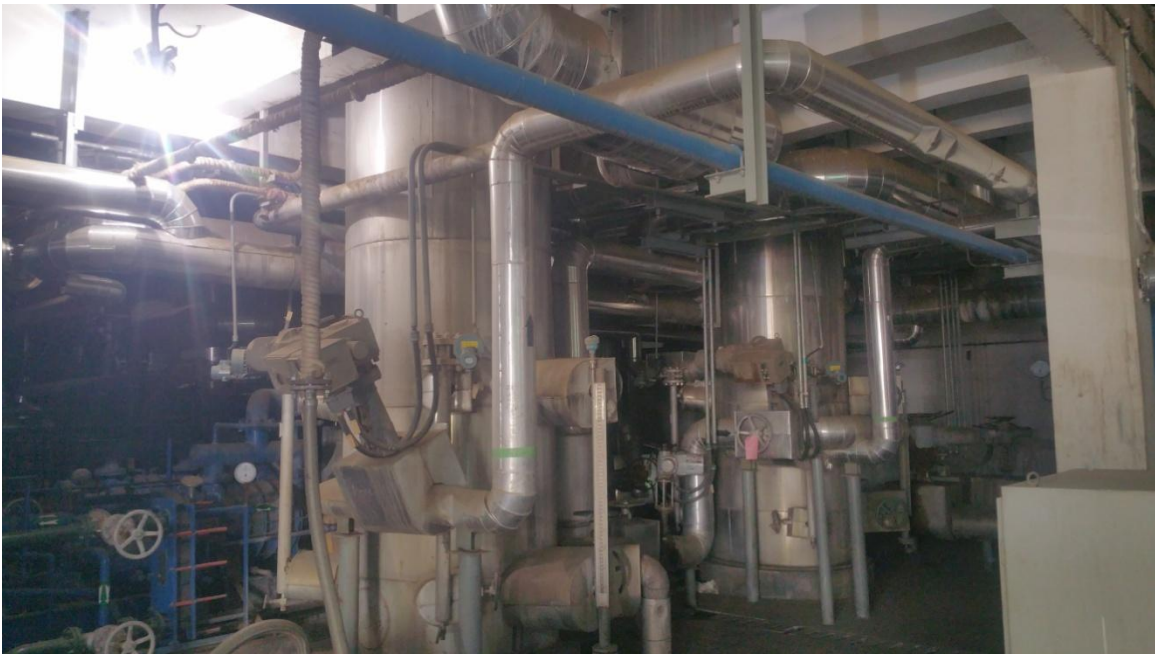
High pressures heaters & valve
