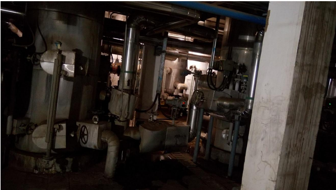
Side water of high pressure heater
