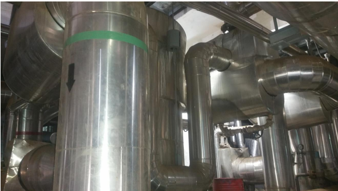
Outlet water of high pressure heater
