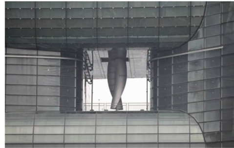
Wind Turbines Mechanical Floor
