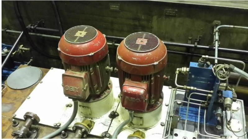
Figure (3.1b) Pressurization Pumps Drivers
