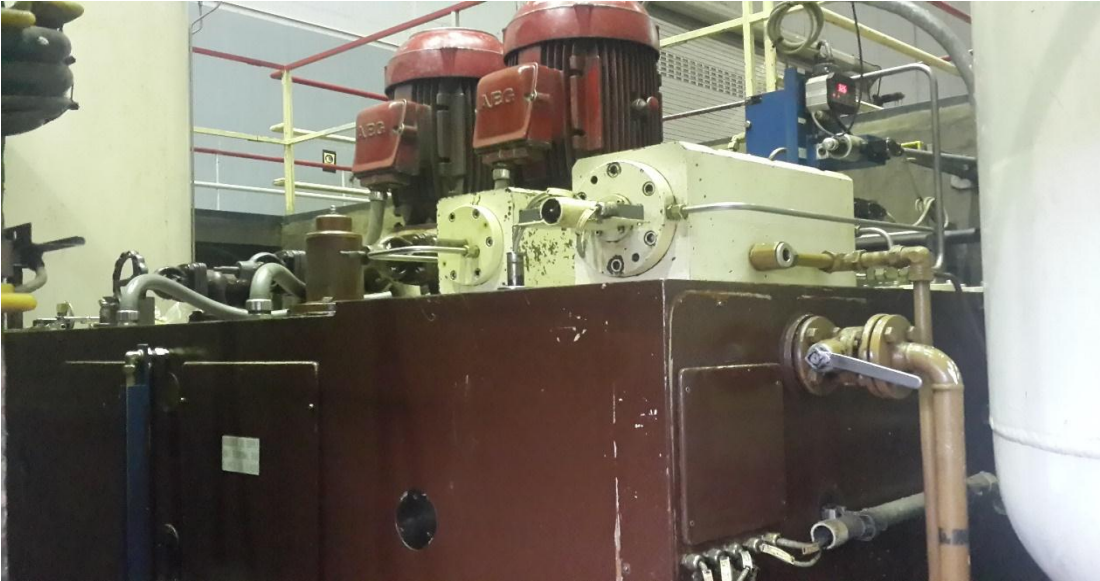
Figure (3.1d) Sump Tank
