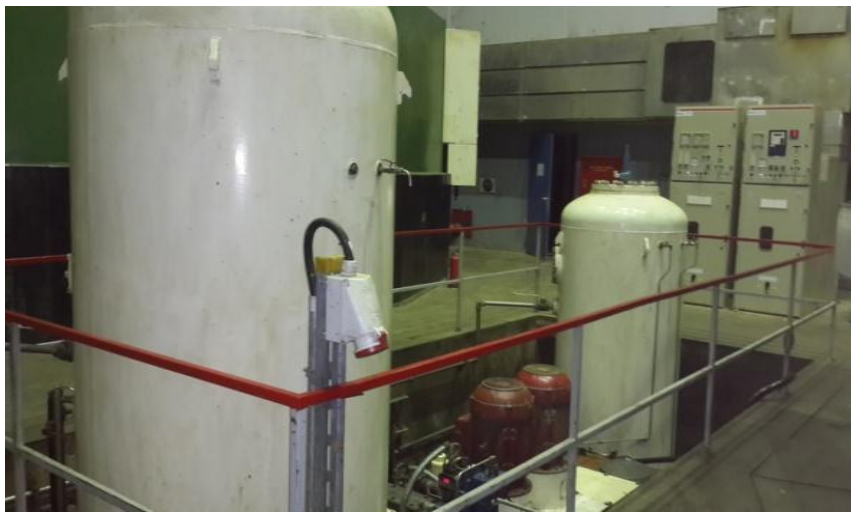
Figure (3.1c) Accumulators
