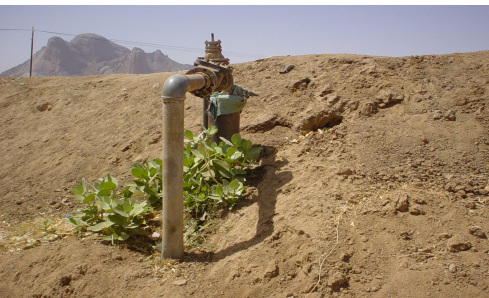
Figure 14: Typical example of undesired activities
