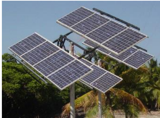
Figure 2.5 Tracking Solar Panel Mount
