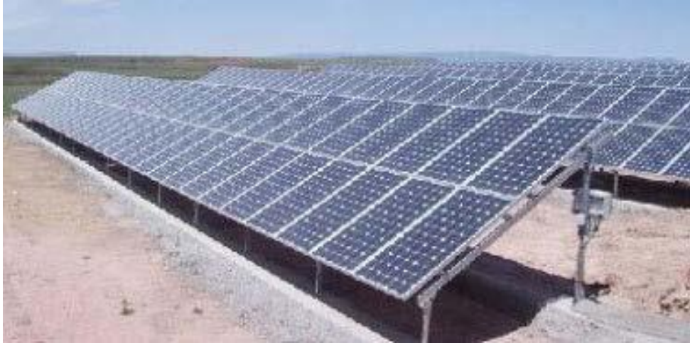
Figure 2.3 Fixed Solar Panel Mount
