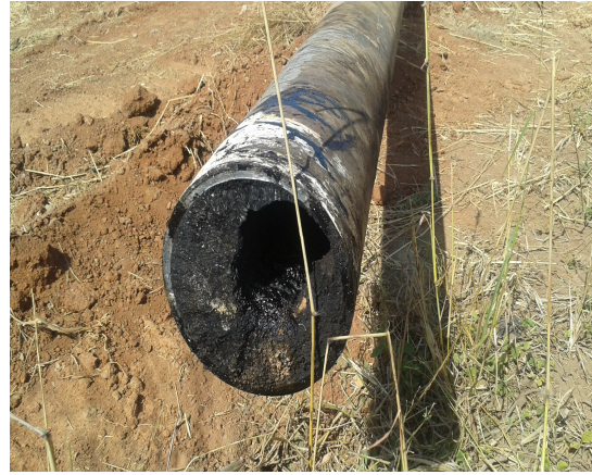
Abandoned pipeline due to heavy scale formation
