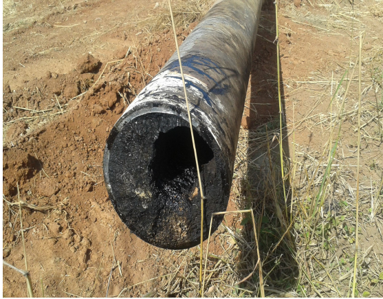
Figure 2-13: An abandoned pipeline due to heavy scale formation
