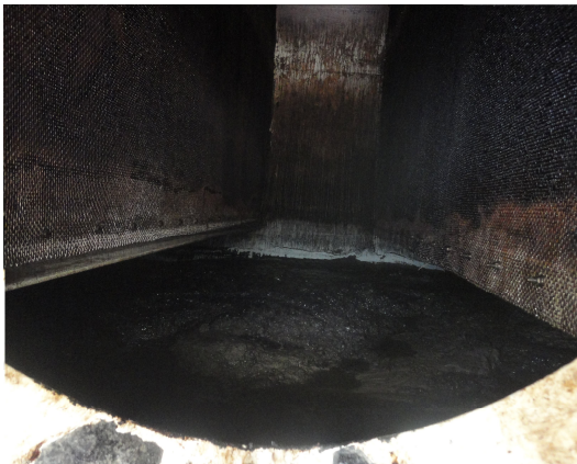
Sludge inside heater treater
