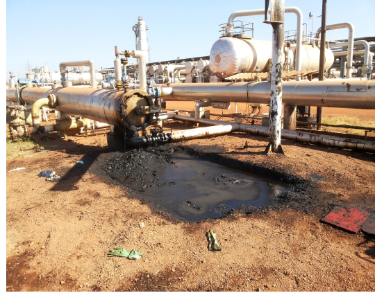
Figure 2-16: Sludge bit at big receiver
