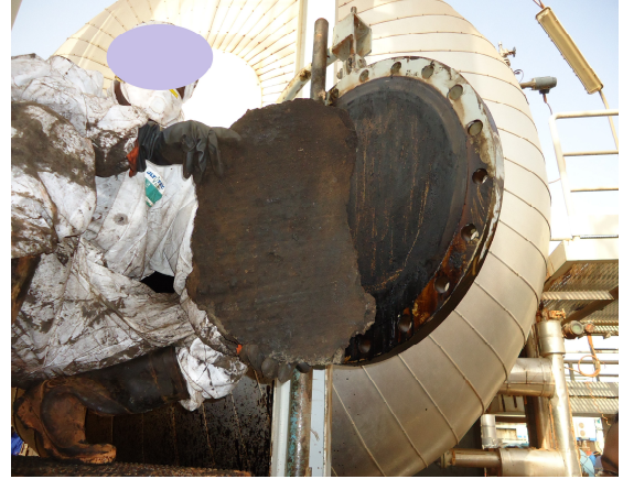
Figure 2-14: A bulk of scale extracted during maintenance
