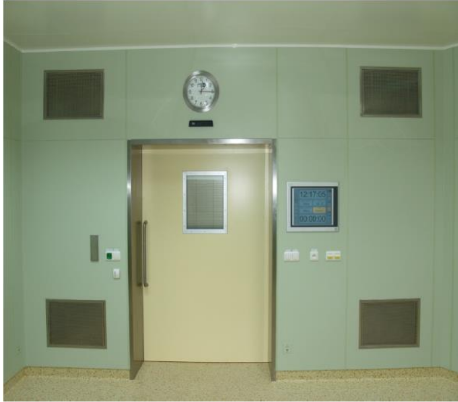
Fig (4.1): ventilation system in operation complex
