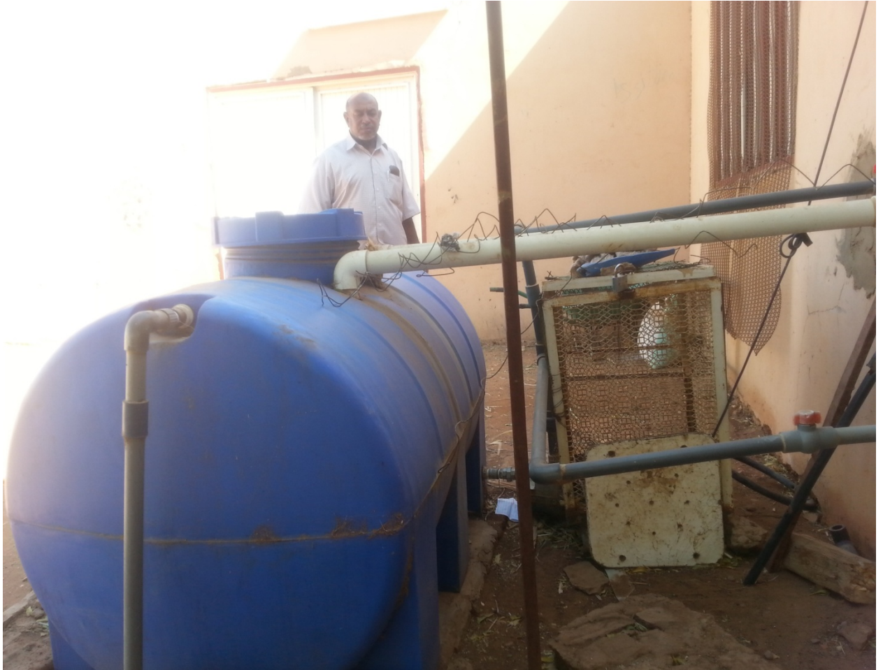
Tank used for storing water for cooling system
